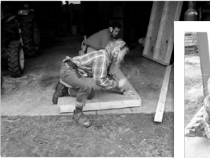
Jim Foxvog and Alex Rodriguez work together on building a new privy/outhouse for the strawberry field
